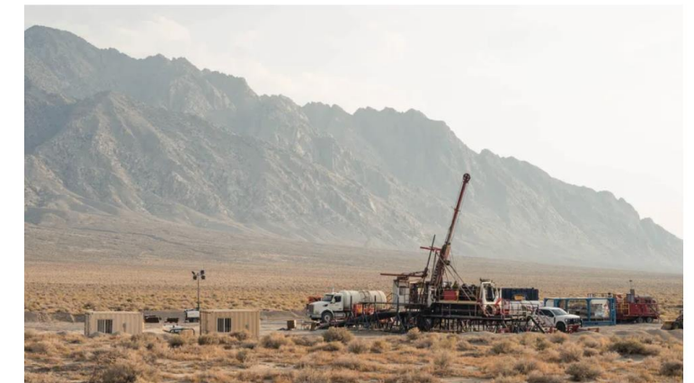
A geothermal drilling rig at Zanskar's new Big Blind site, located in rural Nevada (Zanskar)
